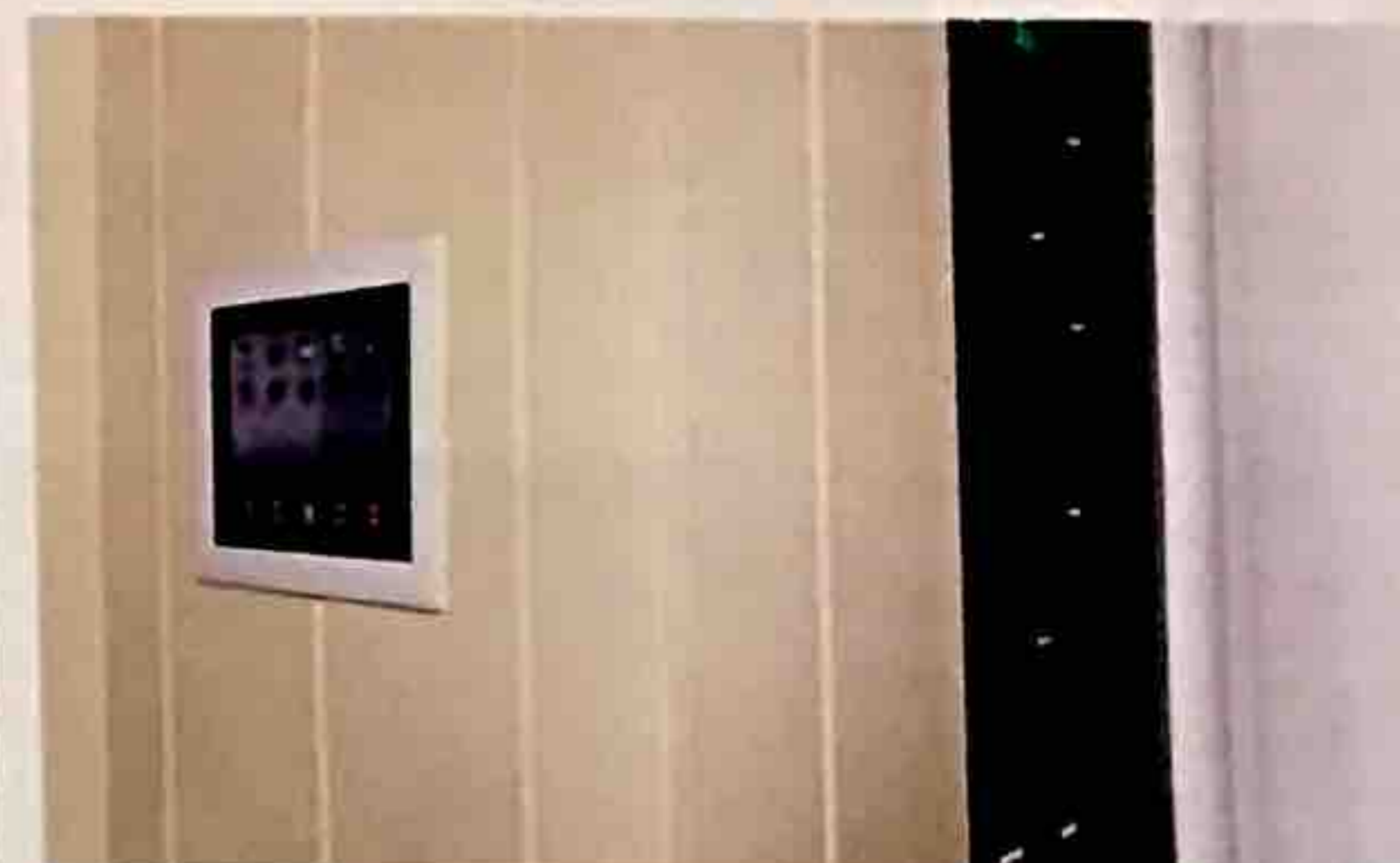
Control a press away and attractively hidden electronics control every aspect of both homes.
